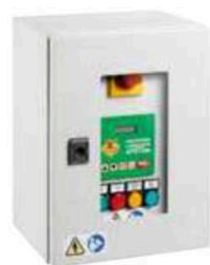
Control equipment (PLC) (page 51-52)
